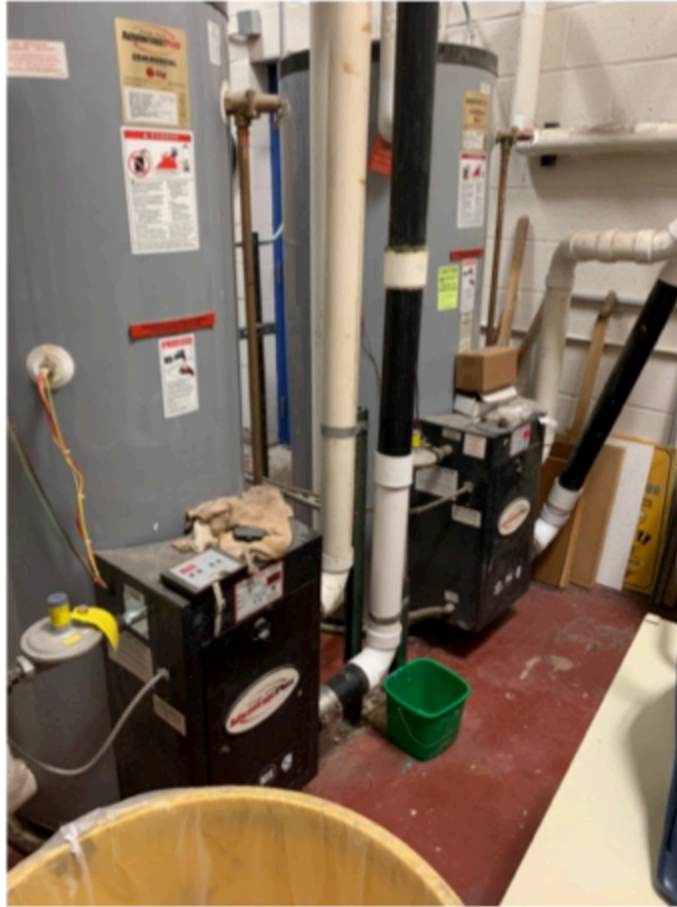
Figure 4 – Domestic Hot Water Heaters
